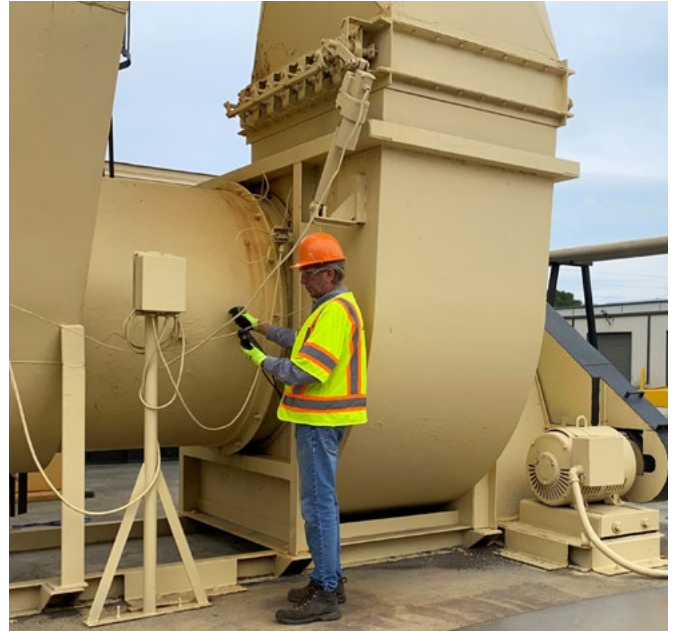
Figure 11. A burner technician measuring exhaust gases through a pre-drilled hole to ensure proper burner tuning
