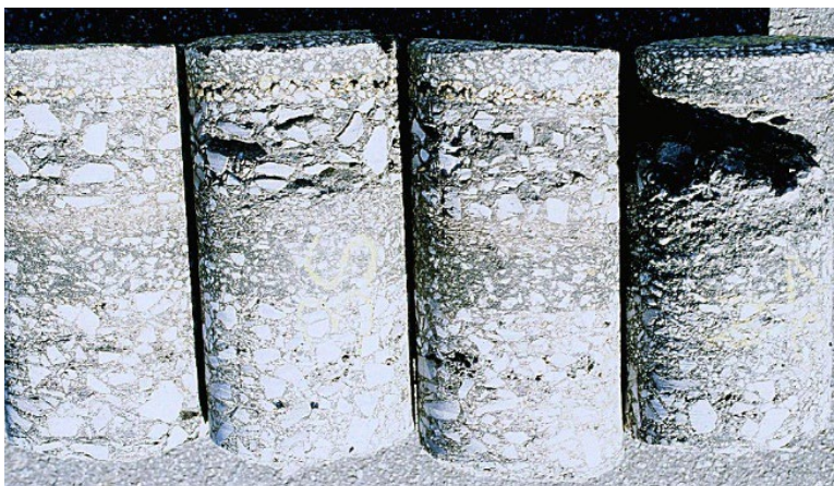
Figure 7. Cores from an Asphalt Pavement Showing Moisture Damage in a Near-Surface Layer.
