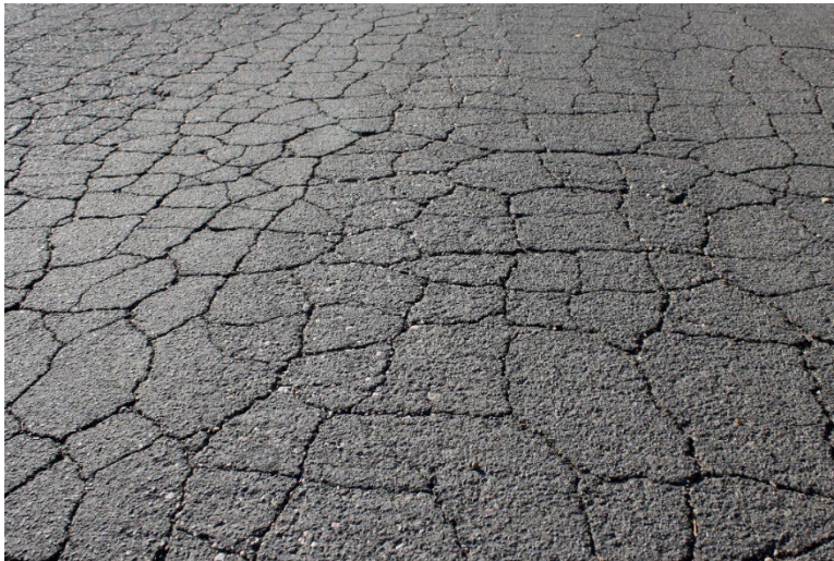
Figure 4. Extensive Fatigue Cracking of an Asphalt Pavement.
