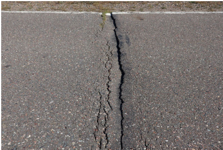
Figure 5. Thermal Crack in an Asphalt Pavement.
