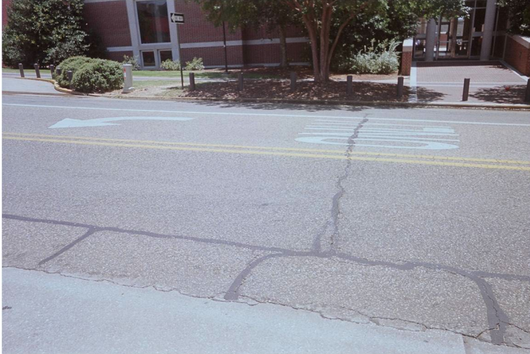
Figure 6. Reflection Cracks in an Asphalt Overlay on a Concrete Pavement.
