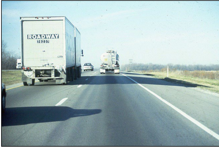
Figure 2. Rutting on an Interstate Pavement.
